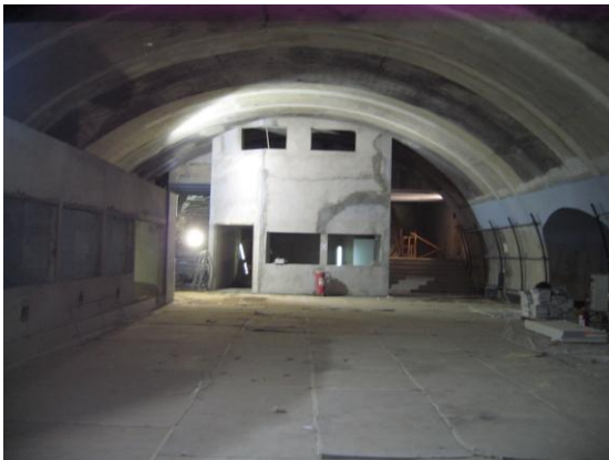
Ticket Hall Analysis of Sealing Problems
